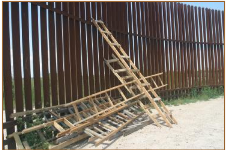
Walls are easily and inexpensively defeated. This photo of a pile of ladders on the south side of the border wall in south Texas proves how easily the wall can be surmounted in a matter of seconds. Photo: Scott Nicol
