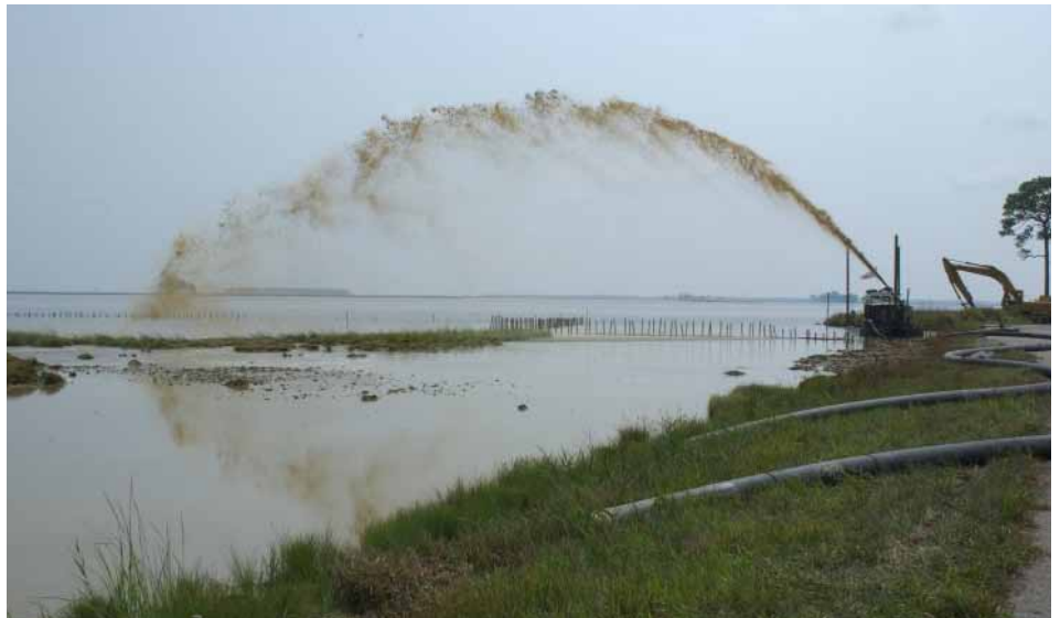
A hydraulic dredge sprays a thin layer of dredged material to restore a wetland at Blackwater. Using dredged sediment from U.S. Army Corps of Engineers channel maintenance operations in Chesapeake Bay to rebuild marshes is promising, but hauling it to the refuge is expensive.
